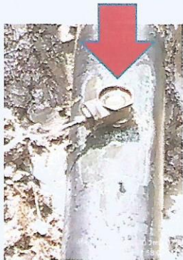
Pic1: Showing one (1no.) 2" valve illegally installed on the pipeline
